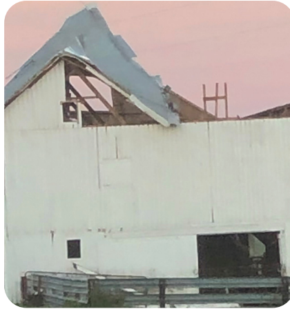
A roof torn from a barn on Maquoketa Valley REC lines.
