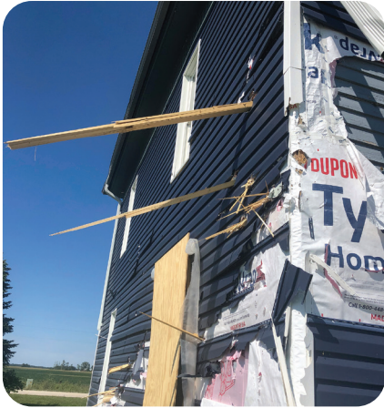
The room was occupied in this home on Linn County REC lines when the 2x4s flew into the house.
